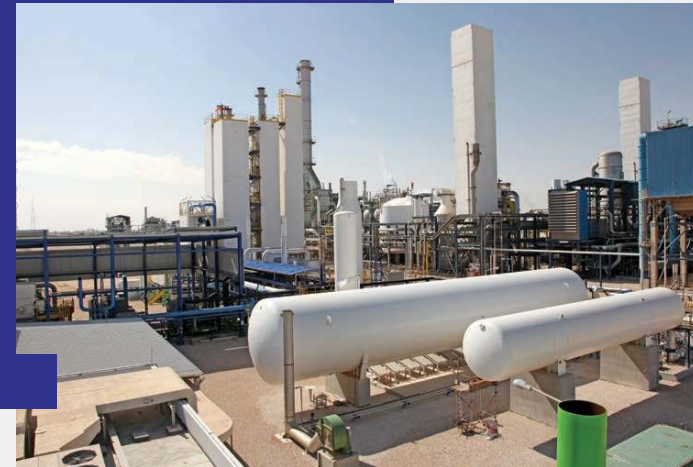
GASAL AIR LIQUIDE AIR SEPARATION PLANT ORYX - RASLAFFAN
